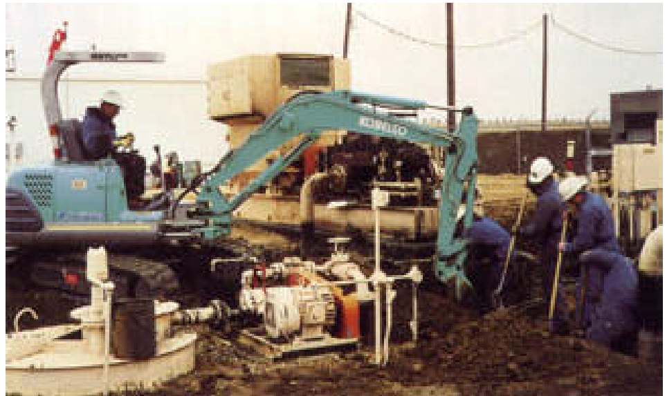
Long's Excavation and Construction, Torrington, Wyoming, depends on its fleet of Kobelco compact excavators for work in tight quarters.
